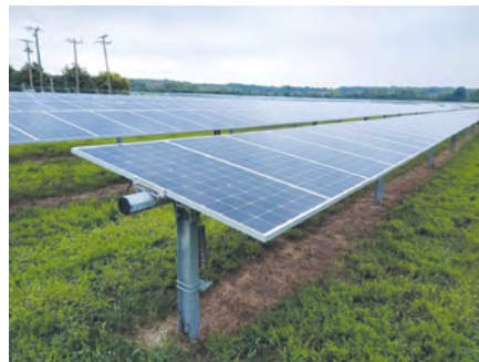
Local 50 continues to support a diverse energy portfolio that contains all forms of generation and fuel types, including solar fields like this one in central Virginia.
